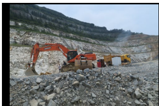
使用機動工具研磨、開鑿、切割或衝擊石塊 The use of power-driven grinding, chiselling, cutting or percussive tools on rocks
