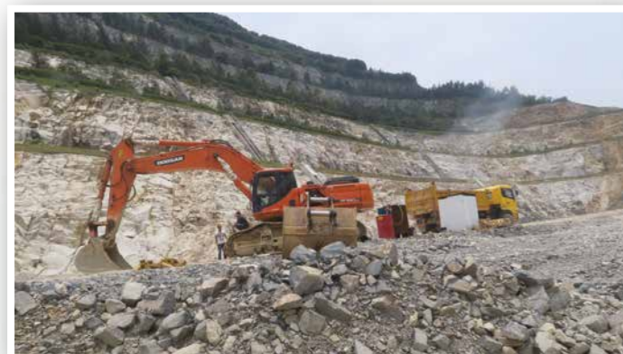
使用機動工具研磨、開鑿、切割或衝擊石塊 The use of power-driven grinding, chiselling, cutting or percussive tools on rocks
